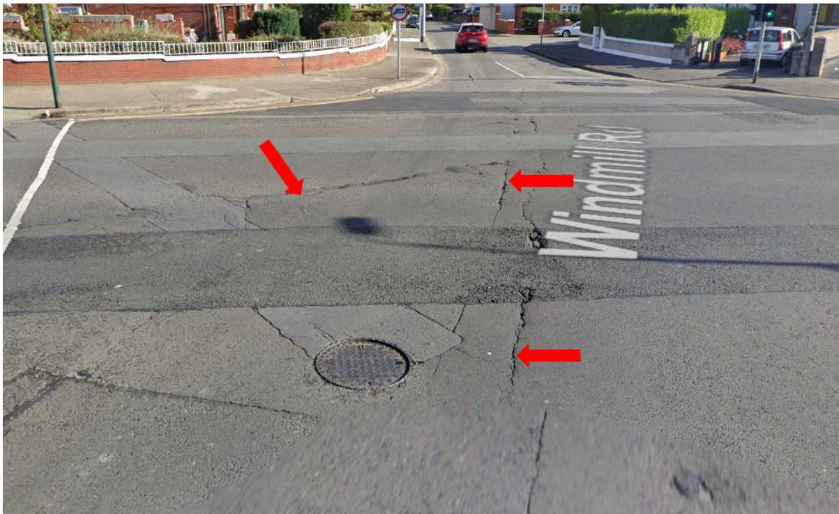
Figure 7-11: Localised Poor Road Pavement Condition at Kildare Road / Windmill Road Junction ©2018 Google Maps
