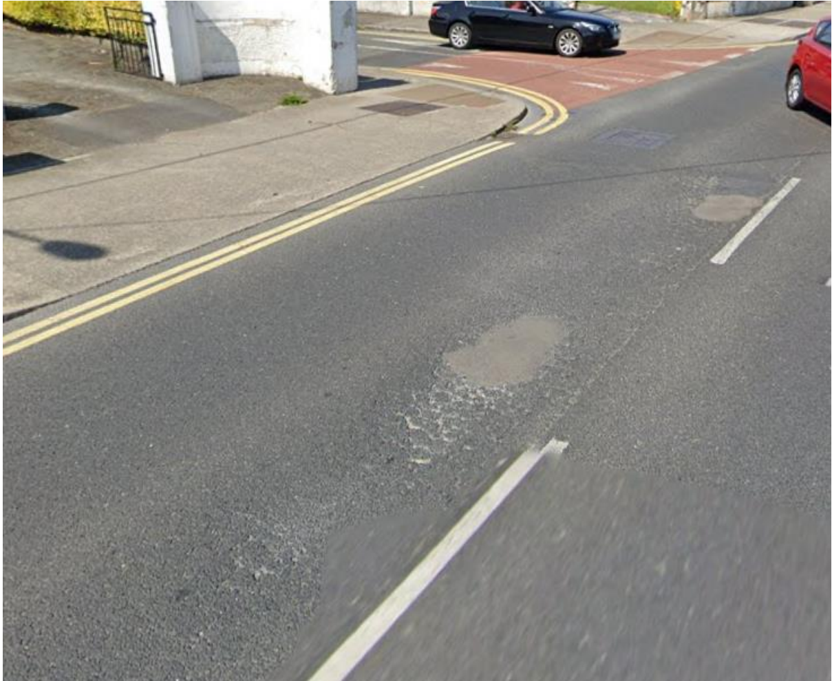
Figure 7-12: Localised Poor Road Pavement Condition at Walkinstown Road / Walkinstown Drive Junction ©2019 Google Maps
